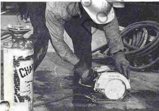
An XL-100 circular saw with Diamond Blade and water attachment is being used here to score a section of pavement which is to be removed.
