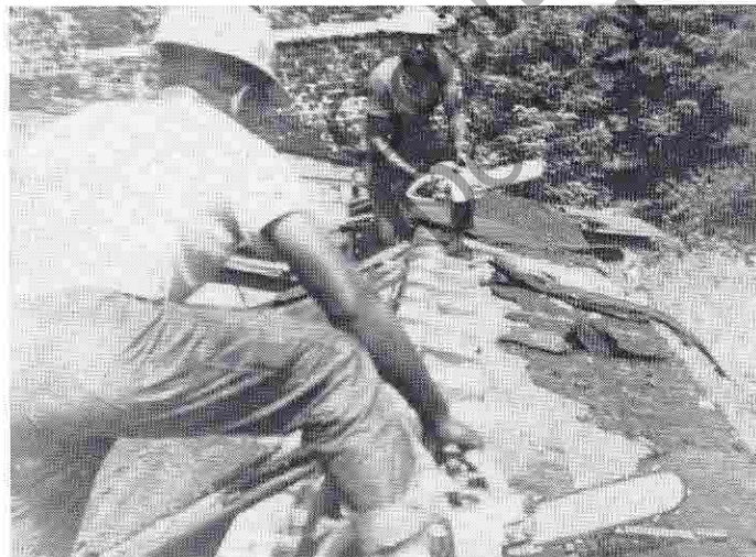
Members of a wrecking crew are shown using XL-12s to cut and remove a large roof on an ice house in Monroe, Louisiana, in less than three hours. Such a job had formerly taken two or more days. The saws were sold by Martin's Engine Service of West Monroe, Louisiana.
